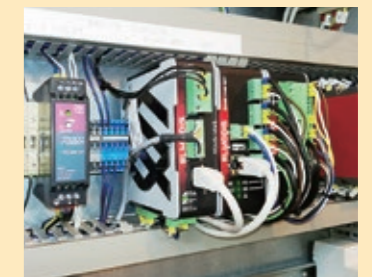
Example of a remote monitoring system installation
