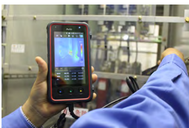
Thermal imaging analysis at walk through
