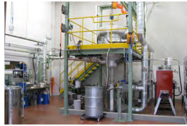
Dissolution plant exterior
