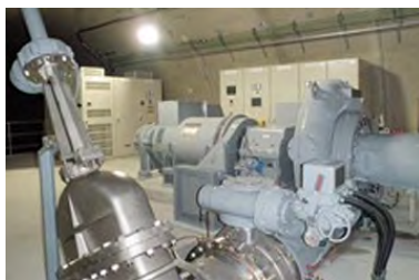
Hydroelectric power generation equipment
