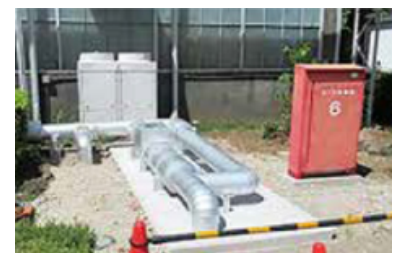
Above-ground water supply pipes
