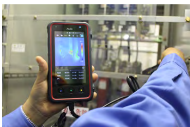
Thermal imaging analysis at walk through
