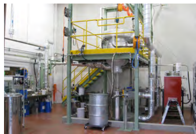
Dissolution plant exterior
