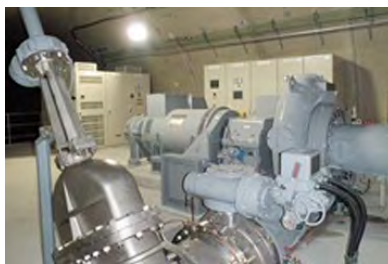
Hydroelectric power generation equipment
