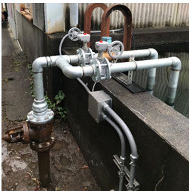
Discharge control valve
