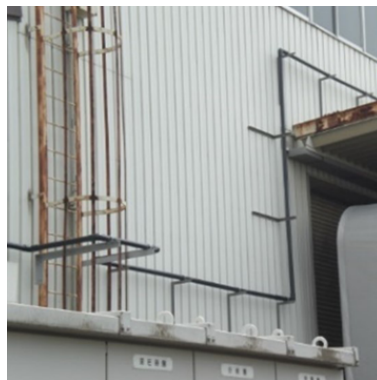
Above-ground industrial water pipes at a factory
