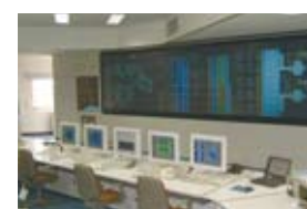
Supervisory control system
