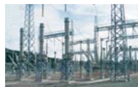
Traction power system
