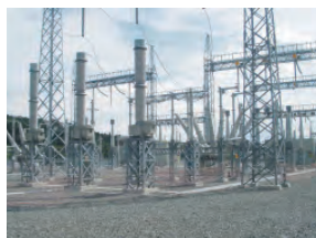
Traction power system
