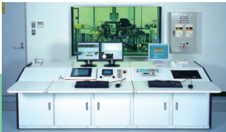
▲ Ono Sokki, operation and measurement, control panels
