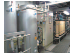
Membrane filtration system for drinking water production
