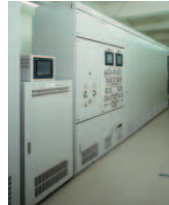
Protection relay and control panel for "Shinkansen line" substations
