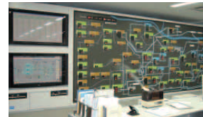
Monitoring and control systems
