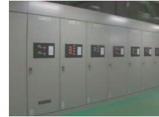
Traction power substation
