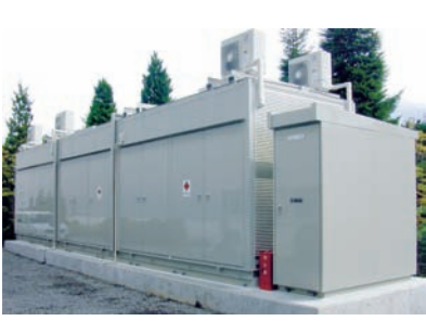
Meiposs-MCP dynamic voltage compensator, high-voltage type (2,000 kVA)
