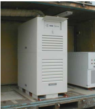
Digestion gas power generating system
