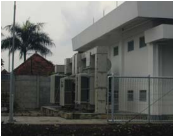
JABOTABEK railway substation
