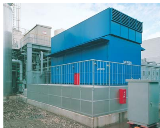
Power conversion system for NAS batteries
