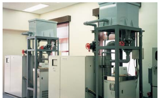
Control system for the disinfection of primary effluent
