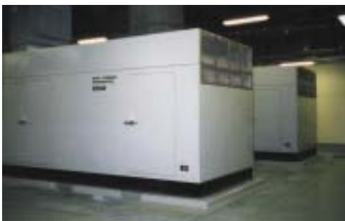
Emergency power generating facility
