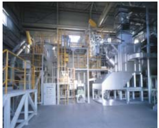
Dry-distillation type thermal decomposition disposal system
