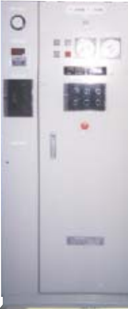
Ozone generating Unit for deodorization
