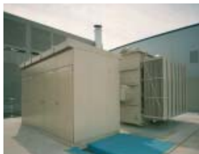
Extra-high voltage power substation facility
