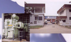
150MVA power transformer
