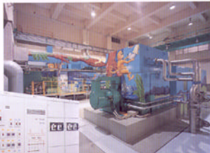
Super Refuse Power Generating Facility
